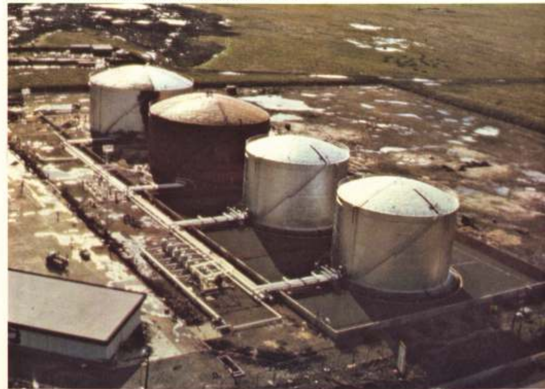
Tank Farm for aviation fuel storage at Nairobi Airport, Kenya.
