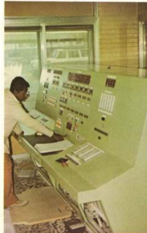
Control console installed for automatic monitoring of product movement through the hydrant system at KAFCO, Kuwait
