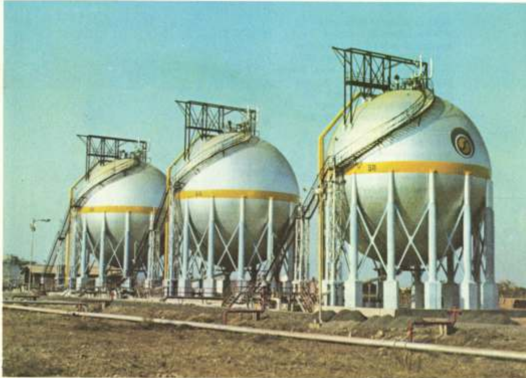
3 nos. 2500 cubic metre LPG Storage Spheres constructed for Bharat Petroleum, in Bombay
