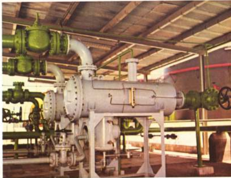
Filter water separators as part of aviation fuelling facility in Hulule, Maldives.
