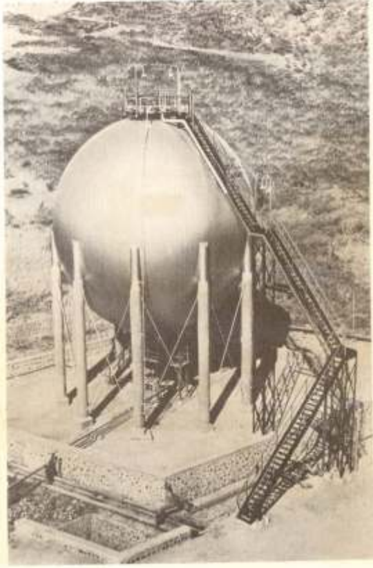
1,350 M 3 high pressure LPG storage sphere at Hindustan Petroleum Corporation
