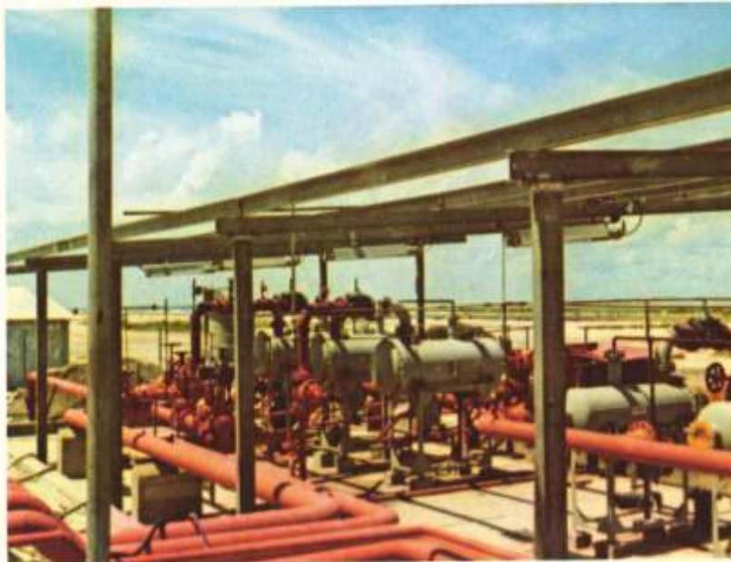
A pump house for an aviation fuelling facility in Hulule, Maldives islands.
