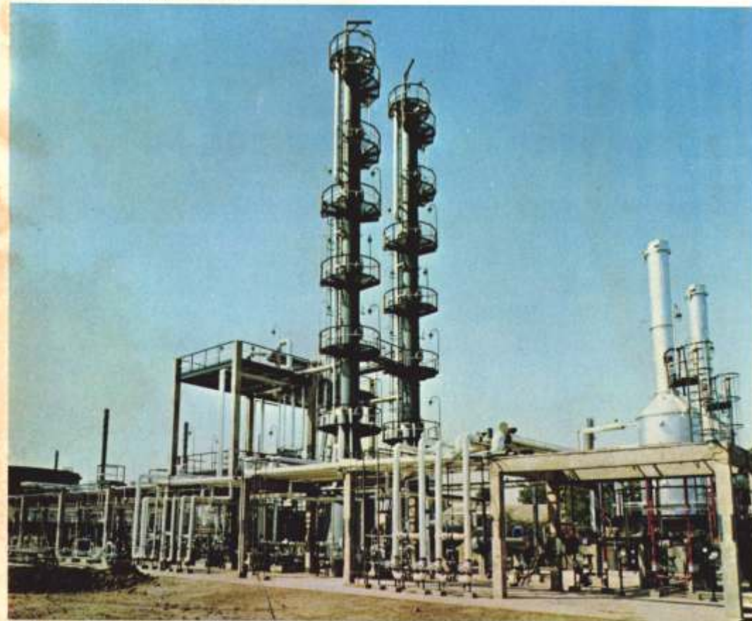
Pilot distillation facilities Plant for Gujarat Refinery to process feedstocks for producing speciality products
