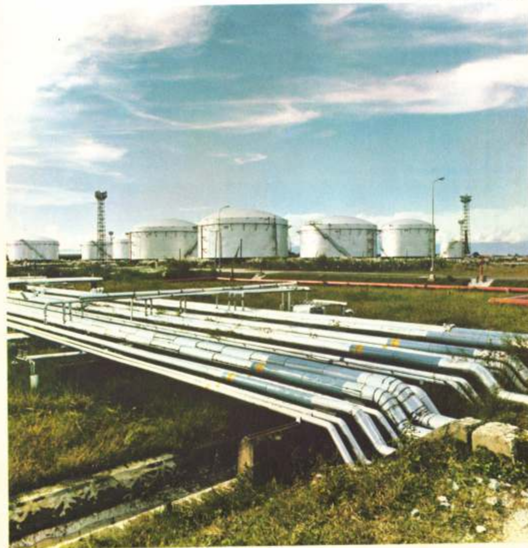
A view of a Tank Farm and Piping in Bongaigaon Refinery where 43 tanks and 80 kms. of piping were constructed
